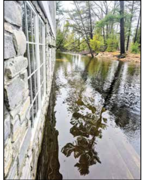
Photo of April flooding at The Mill on the Crystal River by Norm Wheeler
